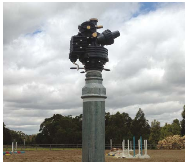
Rotor ST-1600-HS-BR instalado
